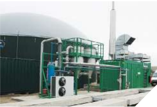
Handewitt, Germany 400 kW CHP in a Biogas plant with gas cleaning system
