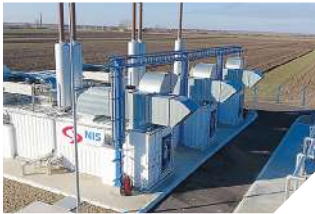
Majdan, Serbia 5 x 500 kW fully containerized power plant
