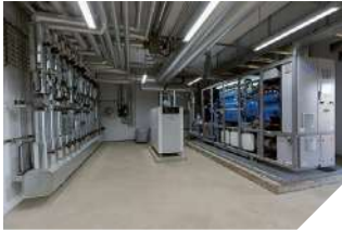
Frechen, Germany 140 kW CHP in an educational institute
