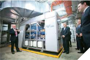
Sydney, Australia 2 x 260 kW CHP to supply the Olympic swimming pool
